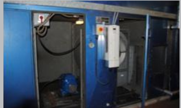
Example 2: Replaced old style fan and installed direct drive AC 'plug fan'
