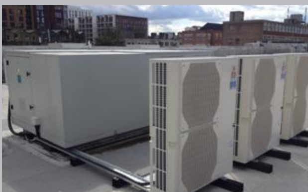
Example 1: Removal of old cooling system and installation of new remote heat pump
